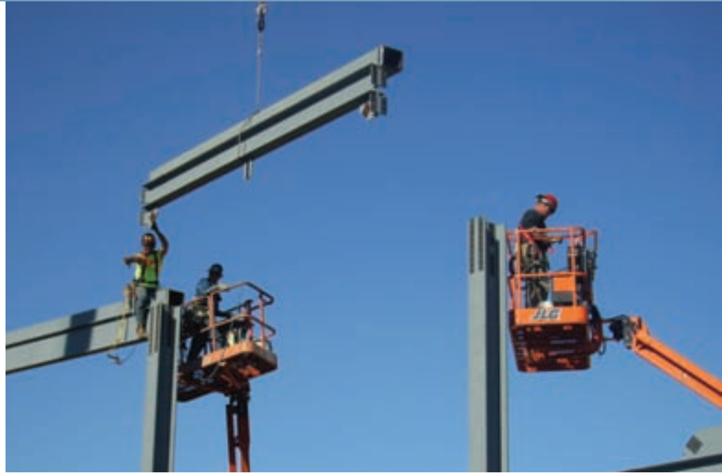
CCB crews erect a steel structure at the new international border crossing station in Calais, Maine.
