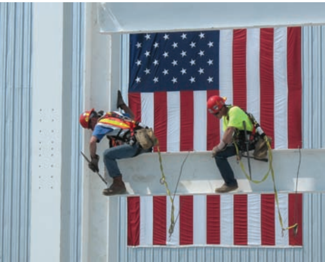
Crane operator Phil Bolduc captured this patriotic image of a CCB crew working at BIW.
